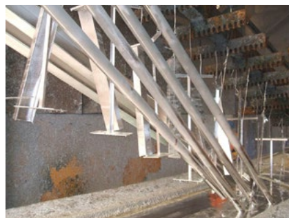
Figure 10: Hot dip galvanized coating on pipe changing to dull appearance while still being withdrawn from the molten zinc.
