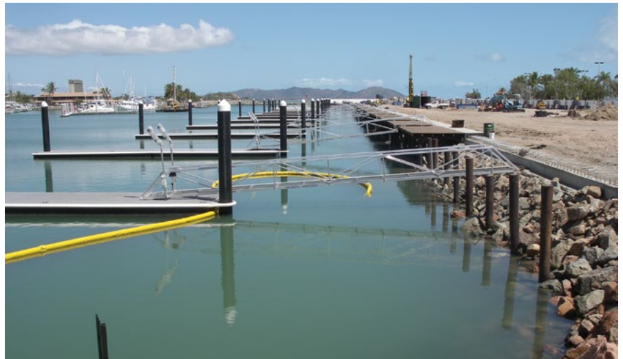
Galvanized rebar was used extensively in the Townsville, Queensland marina.
