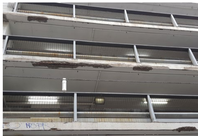
A multi-storey car park suffering from spalled concrete due to corrosion of the rebar
