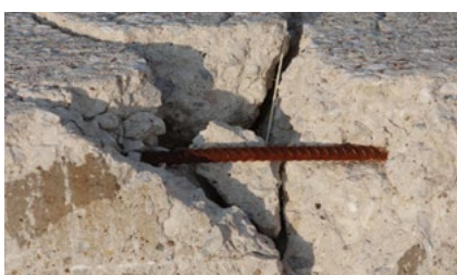
An example of galvanized and uncoated steel reinforcement exposed in a bridge after damage from an earthquake. The uncoated bar has begun to corrode while the galvanized reinforcement is still in excellent condition
