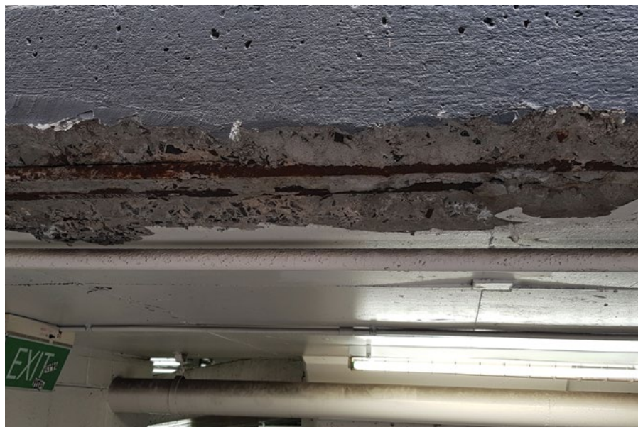
Cracking and spalling of cover concrete due to corrosion of the reinforcing steel
