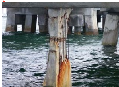
Reinforcement and concrete failure in a high chloride (coastal) environment
