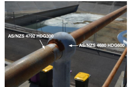
The handrail above was about 7 years old in a C5 wastewater treatment and marine environment when the photo was taken. The post was hot dip galvanized to AS/NZS 4680, while the rail was produced to AS/NZS 4792 HDG300 – or about half the nominal coating thickness of the post. The weld joining the rails was never repaired. Clearly, the after fabrication galvanized post to AS/NZS 4680, with at least double the original coating thickness of the continuously galvanized rail to AS/NZS 4792, has provided superior corrosion protection of the base steel.
