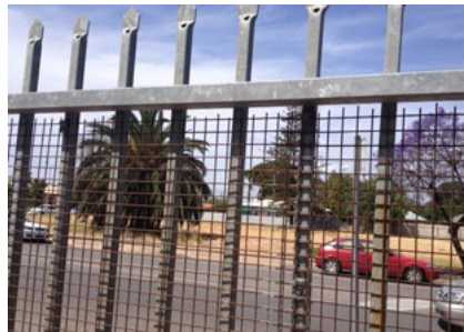
The same fence from another angle, showing the galvanizing on the wire mesh has broken down and rust has stained the entire structure, while the tubular after-fabrication galvanized fence is still rust free.
