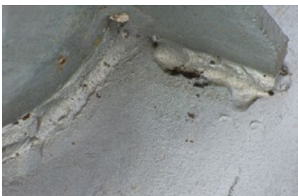
Figure 1: Poor welding practice can lead to areas of uncoated steel and result in surface conditions that collect moisture and detritus both leading to a reduced service life
