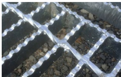
Figure 5: Small weld splatter inclusions can be seen under the galvanized surface. In this case the end use wasn't affected as the weld splatter is strongly adhered to the steel
