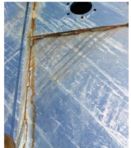
Figure 12: Rust bleeding (staining) from overlapping sections with less than a 2.5 mm gap between stitch welds. This can be remedied after galvanizing through cleaning of the stains and application of a sealant such as silicone in the affected areas
