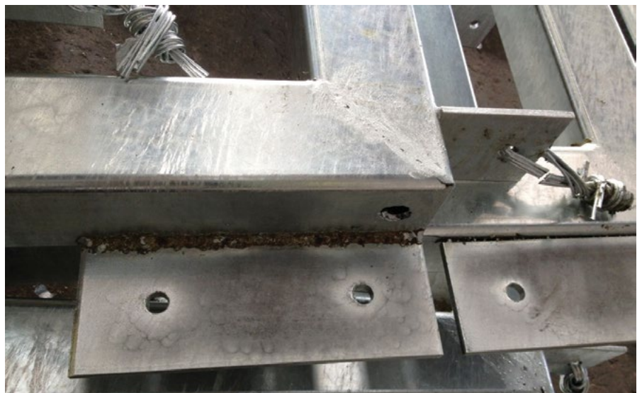
Figure 7a: Welding slag hasn't been cleaned by the fabricator after welding and has created a bare spot
