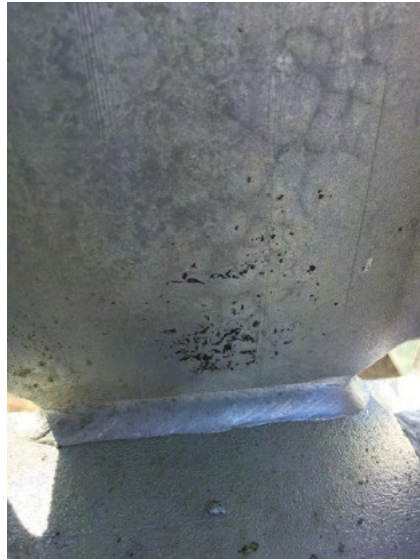
Figure 6: In this case an oil-based anti-spatter spray hasn't been cleaned off by the fabricator prior to galvanizing and has created a series of small bare spots
