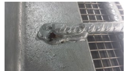
Figure 2: A porous weld has allowed pre-treatment solutions to become trapped inside, resulting in a bare spot near the weld
