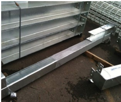
Figure 9: While not a welding defect, steels of different compositions that have been welded together in the same plane prior to galvanizing can result in a differing appearance after hot dip galvanizing
