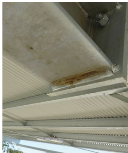
Figure 11: A weeping weld causing rust staining around the weld surface as the corrosion products reach the surface
