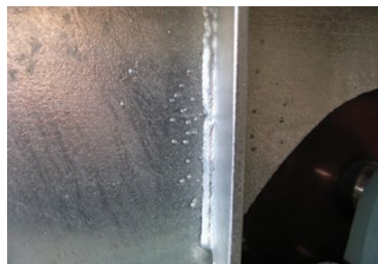
Figure 4: Weld splatter inclusions are usually spherical due to the surface tension of the metal while molten. They are often highly adherent and may not affect the corrosion protection, but are always a problem when the steel is to be subsequently painted or powder coated
