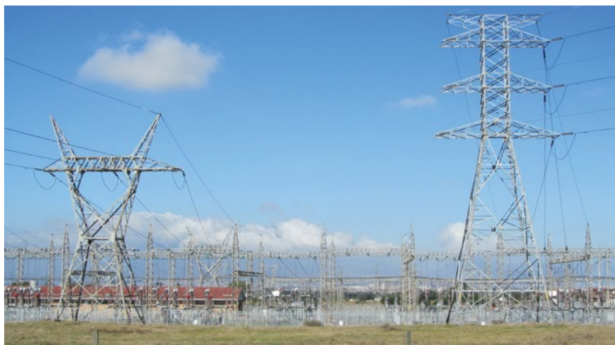
Figure 8: Electrical transmission towers use large numbers of bolted connections for ease of construction and low maintenance in critical infrastructure
